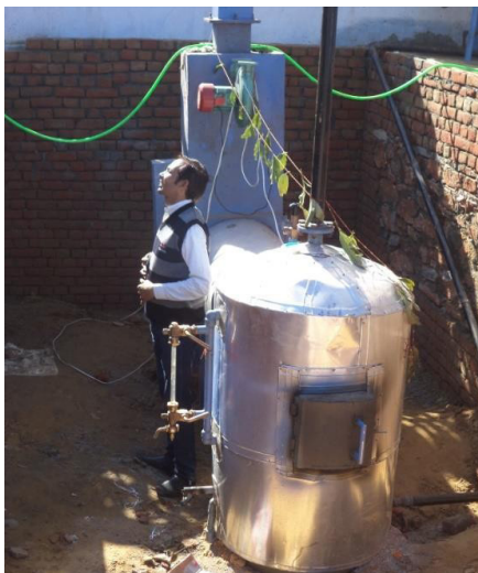
Modified boiler with steam-recycling, installed at a food processing unit by Subhash Ola, Alwar, Rajasthan.
